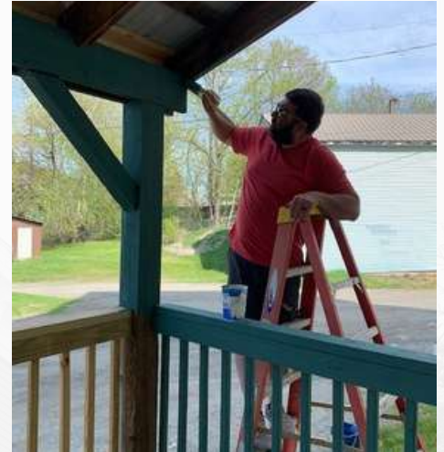
Maintenance Supervisor, Chad McCormick, paints the deck at The Pierce Block as part of RuralEdge's Employee Work Day.
